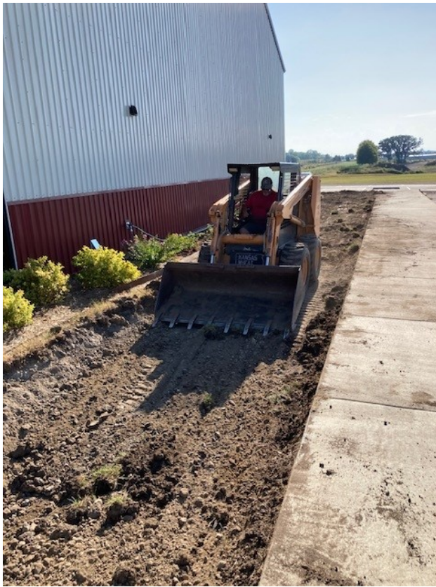
Removing the rubble with the skid loader. It took about 80 cubic yards to backfill the removed materials.
